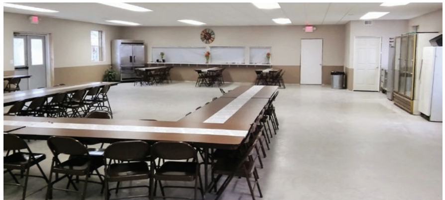
Dining Hall's new look after installing furnace, air conditioning, insulation and drywall. Now ready for trim and chair rail.
